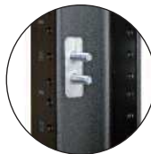
Ground Studs located directly on rack channel
