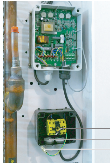
Fig. 30: Electrical connection on the external condenser
