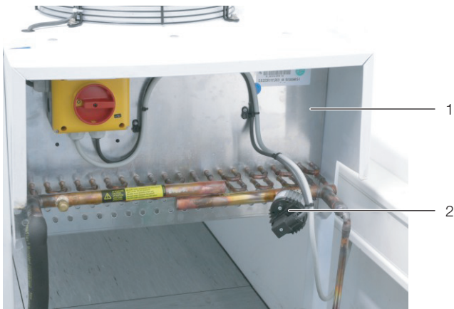
Fig. 25: Pressure switch on the condenser
