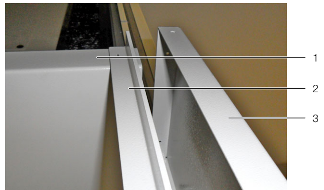
Fig. 53: Roof bracket above the aisle containment door
